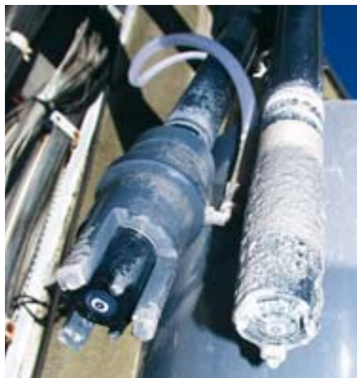
Efficient compressed air cleaning put into practice:
